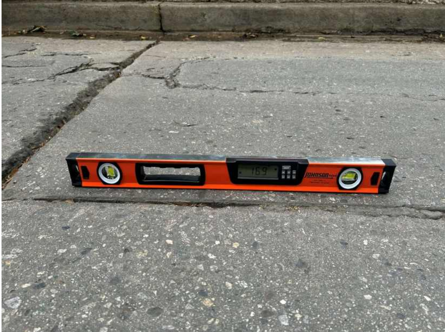
Exhibit 3.1: Photograph 1 of Grade in Excess of 16 Percent Taken Along the Segment of Stanley Hills Drive from Station 0+10.65 to Station 1+64.43
