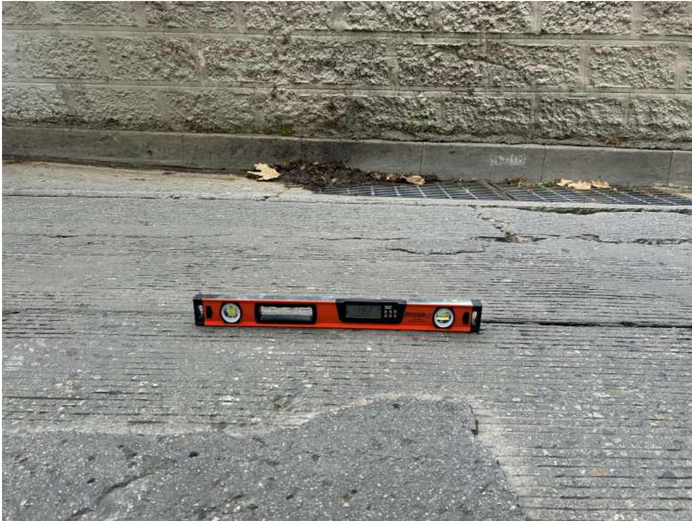
Exhibit 3.2: Photograph 2 of Grade in Excess of 16 Percent Along the Segment of Stanley Hills Drive from Station 0+10.65 to Station 1+64.43
