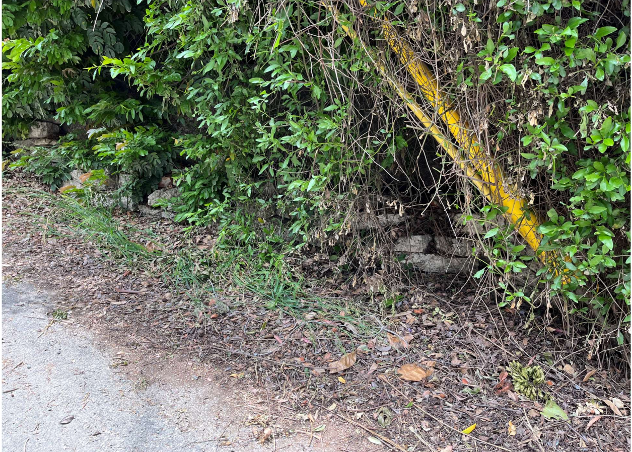
ANOTHER SMALL RETAINING WALL OPPOSITE FROM FRONT ENTRANCE TO 855 N. BEVERLY GLEN BLVD., LA, CA 90077, WHICH COULD POTENTIALLY BE DAMAGED/DESTROYED FROM THE CONSTRUCTION VEHICLES AND TRAFFIC VOLUME.
