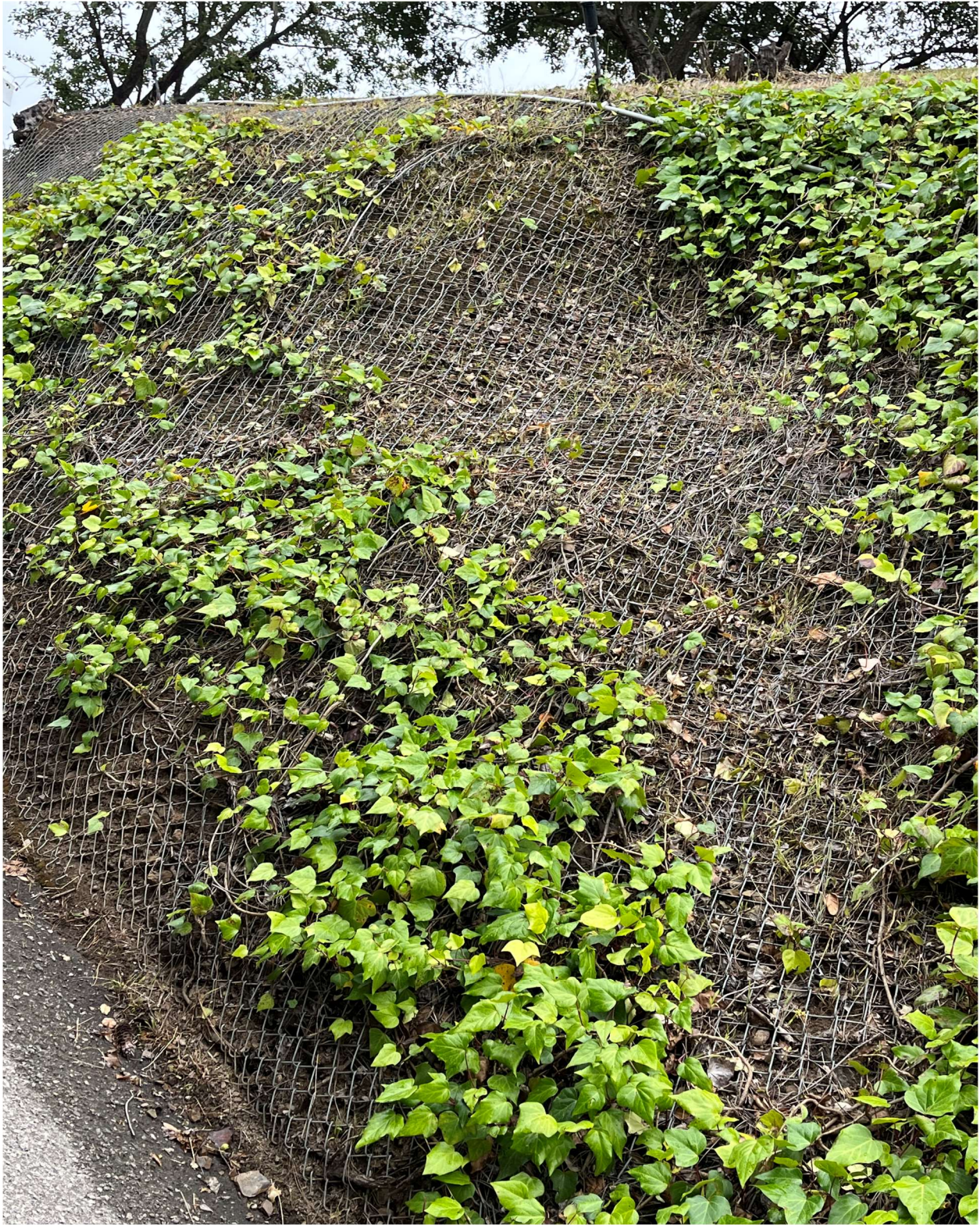
ONE MORE VIEW. AGAIN, THIS CONSTRUCTION WAS MANDATED BY THE CITY OF LA. WITH RESPECT TO 863 N. BEVERLY GLEN BLVD.
