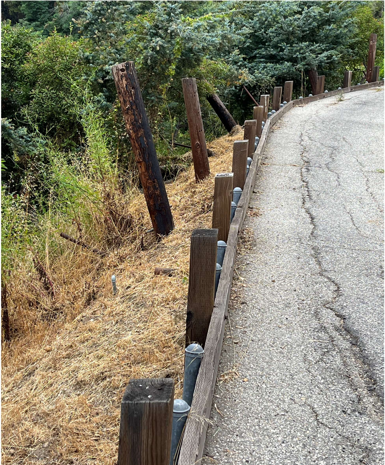
ANOTHER VIEW OF THE PILE-ONS AND THE FRAGILITY OF THE HILLSIDE SUPPORT AND POTENTIAL DAMAGE OR COMPROMISE TO THE HILLSIDE SUPPORTING THE PRIVATE DRIVE/EASEMENT
