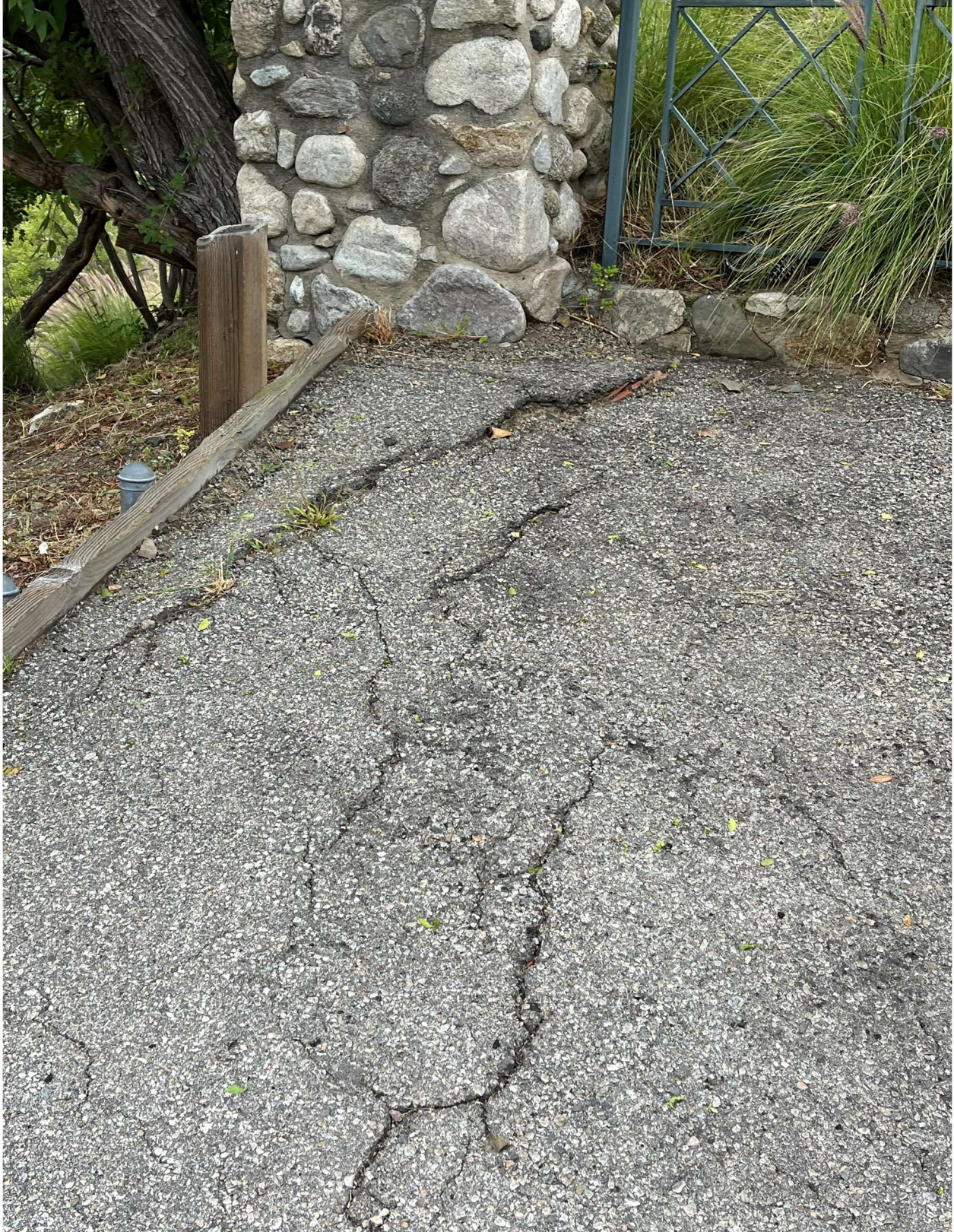
ANOTHER VIEW OF THE CRACKING AND SLIGHT SLIPPING THAT HAS OCCURRED.
