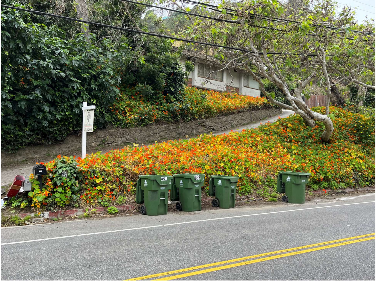
ANOTHER VIEW/PERSPECTIVE OF THE RETAINING WALL/HILLSIDE AND TREES SUPPORTING THE RESIDENTIAL HILLSIDE AND PRIVATE DRIVE/EASEMENT FROM IMMEDIATELY ACROSS THE STREET ON THE EAST SIDE OF N. BEVERLY GLEN BLVD.
